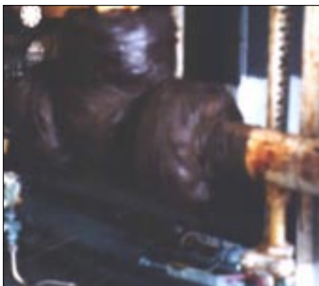
Cocooning system prevents inspection
