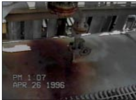
Leaking flange affecting surrounding areas
